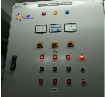
350KVAR Capacitor Panel
