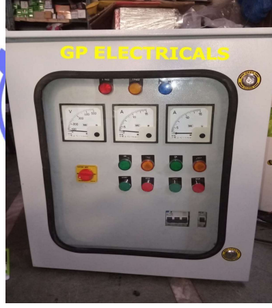
DOL Starter Control Panel
