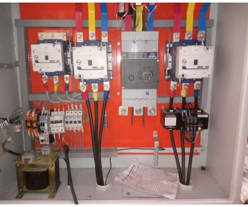
200HP Star-Delta Control Panel
