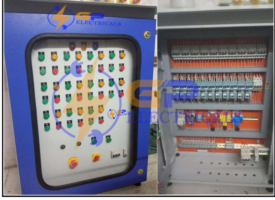
VIBRATOR MOTOR CONTROL PANEL
