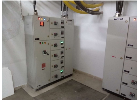
MAIN POWER DISTRIBUTION CONTROL PANEL
