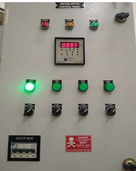
25KVAR APFCR Control Panel
