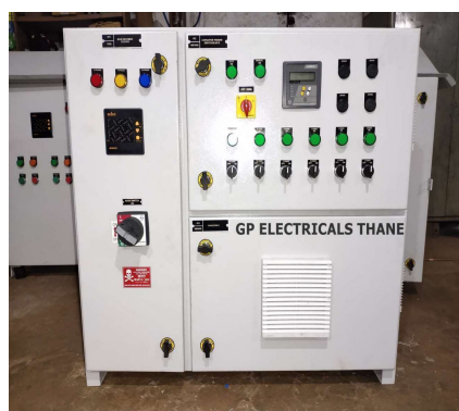
60KVAR APFCR CONTROL PANEL
