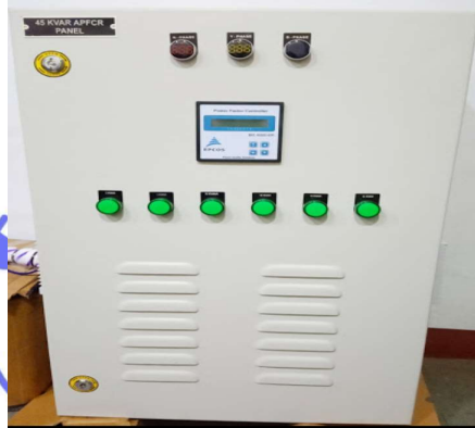
45KVAR APFCR Control Panel
