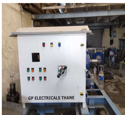
HYDROJET MACHINE CONTROL PANEL
