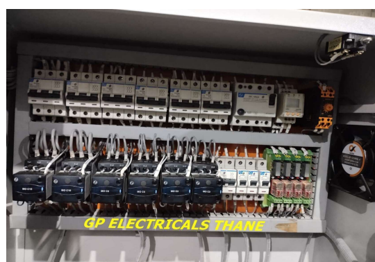
60KVAR APFCR CONTROL PANEL
