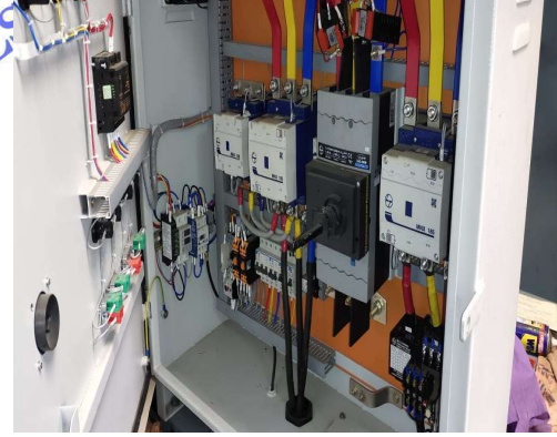
180HP Star-Delta Control Panel
