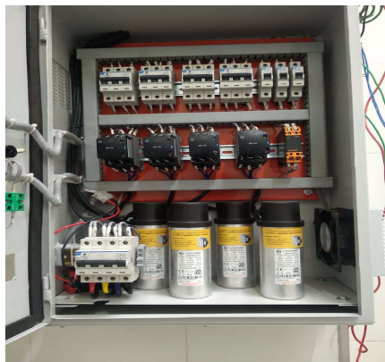
35KVAR Capacitor Panel
