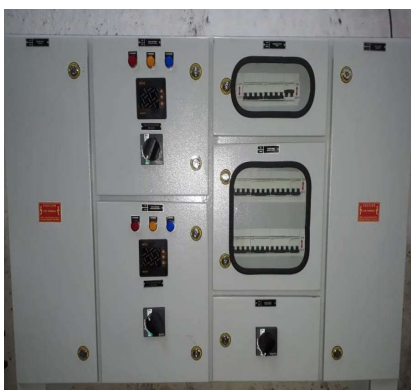
POWER DISTRIBUTION CONTROL PANEL
