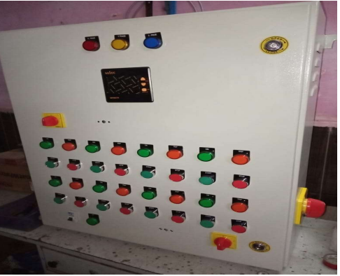
DOL Starter Control Panel
